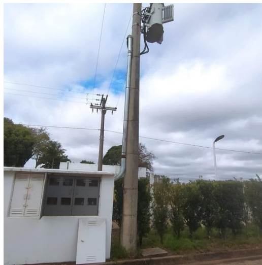
Vista geral – Quadro Principal
