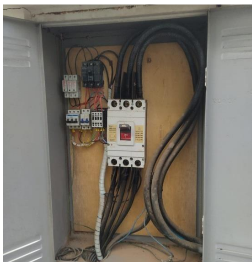
Disjuntor Geral Principal – 300A
